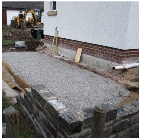
A bedding layer of stone provides a stable level base for the rainwater storage units.
