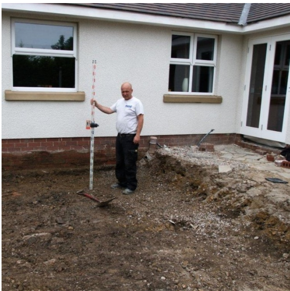
Excavation is less than 500mm, you can see the stain of the original ground level on the wall behind Mark.
