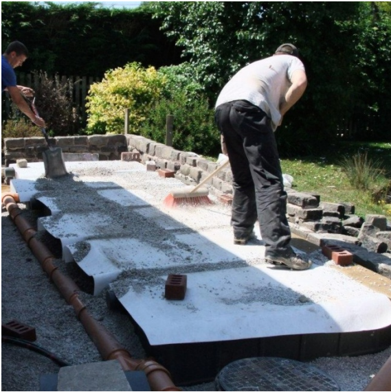
The rainwater storage units are covered with geotextile which comes supplied with the units and a final layer of stone is laid over the rainwater storage units on to which the paving slabs of the patio were laid.
