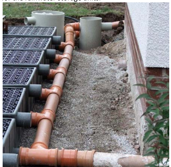
The rainwater storage units are connected together using standard 110mm diameter underground drainage unit.
